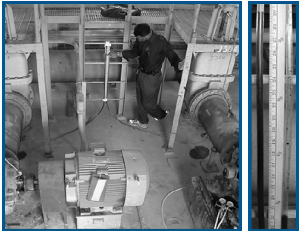
Photo 1 (above left). General layout of pump installation.
