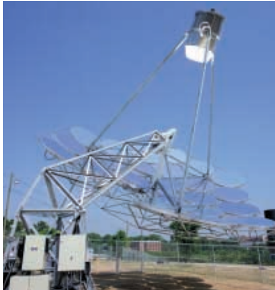
This solar thermal dish/Stirling system was located on a busy pedestrian thoroughfare close to the Olympics Natatorium. The unit, rated at 7 kW, provided electricity to the local electricity grid.
