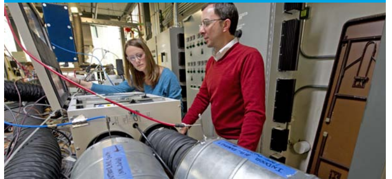
Researchers accurately monitor the nation's emerging efficiency products for indoor comfort at the Advanced HVAC Systems Laboratory. Photo by Dennis Schroeder, NREL/PIX 20008
