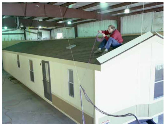
Ron Judkoff gets a bird’s eye view of modular housing efficiency in 1995. Photo by Warren Gretz, NREL 00962
