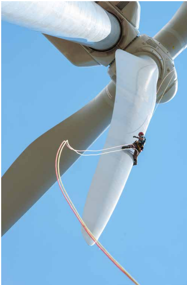
Pete Johnson of Gemini Rope Access Solutions inspects the blade of a 3-MW Alstom wind turbine by rappelling down the blades in August 2013 at the National Wind Technology Center. Photo by Dennis Schroeder, NREL 27196
