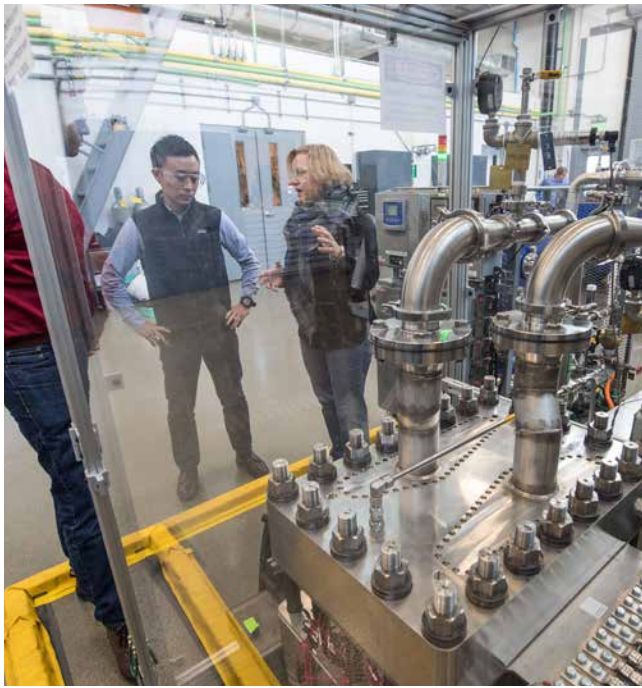
Jen Kurtz (right) talks with colleagues Kazunori Nagasawa and Rishabh Jain in October 2019 while looking at an electrolyzer in the Energy Systems Integration Lab at the ESIF. Photo by Dennis Schroeder, NREL 60020
