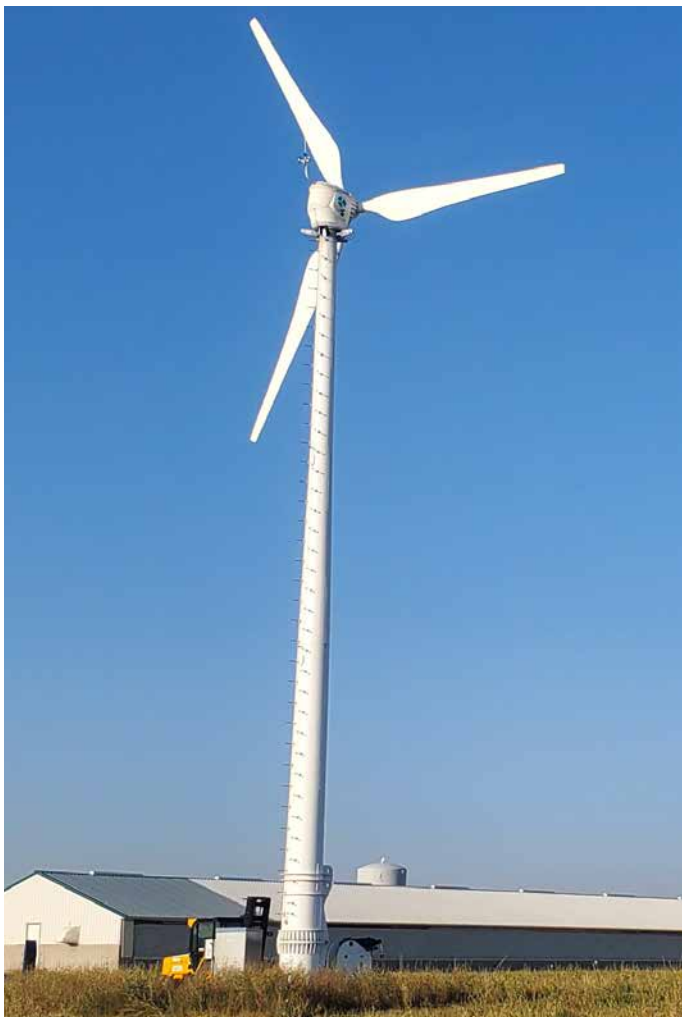
An Eocycle EOX S-16 turbine installed at U.S. food company Smithfield Foods. Photo from Eocycle
