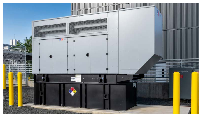
A 540-gallon (2,006-L) diesel AST containing diesel was installed at the newly constructed Research and Innovation Laboratory on the STM Campus to support laboratory growth. Photo by Werner Slocum, NREL 80091
