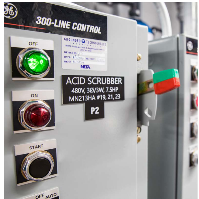
An acid scrubber system in the Science and Technology Facility on the STM Campus helps remove contaminants from exhaust streams. Photo by Werner Slocum, NREL 55971
