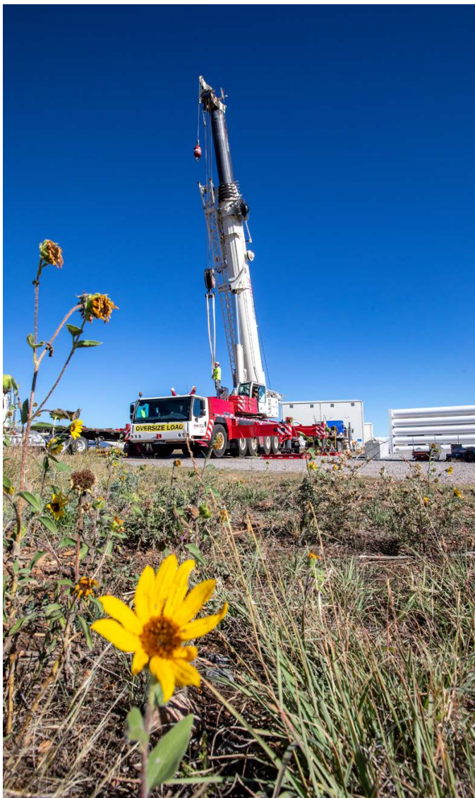
NREL crews and subcontracted crane operators work to install a 1-megawatt fuel cell at the Flatirons Campus. Before outdoor project activities took place, environmental impacts were assessed and communicated so proper environmental protection actions could be implemented. Photo by Werner Slocum, NREL 72220
