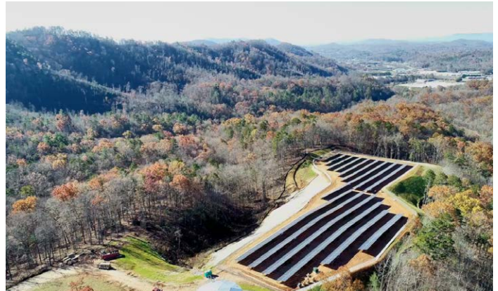
A 705-kW solar array installed near the EBCI-owned casino in Murphy, North Carolina. Photo by Joey Owle, Eastern Band of Cherokee Indians
