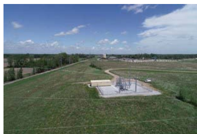
Saginaw Chippewa Indian Tribe of Michigan’s substation supporting Tribal utility operations. Photo by Brian Smith, Saginaw Chippewa Indian Tribe of Michigan
