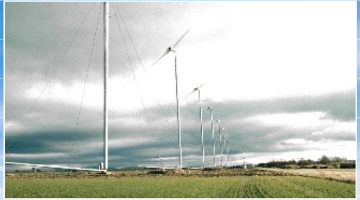
Ten Carter Wind Model 300 wind turbines installed at the Great Orton Wind Farm in 1993 near Cumbria England. Photo courtesy of Carter Wind Turbines.
