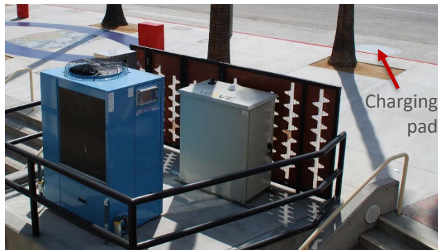
WAVE charging system at the Convention Center
