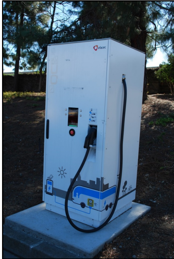
Figure 2-3. Plug-in charger at the County Connection facility
