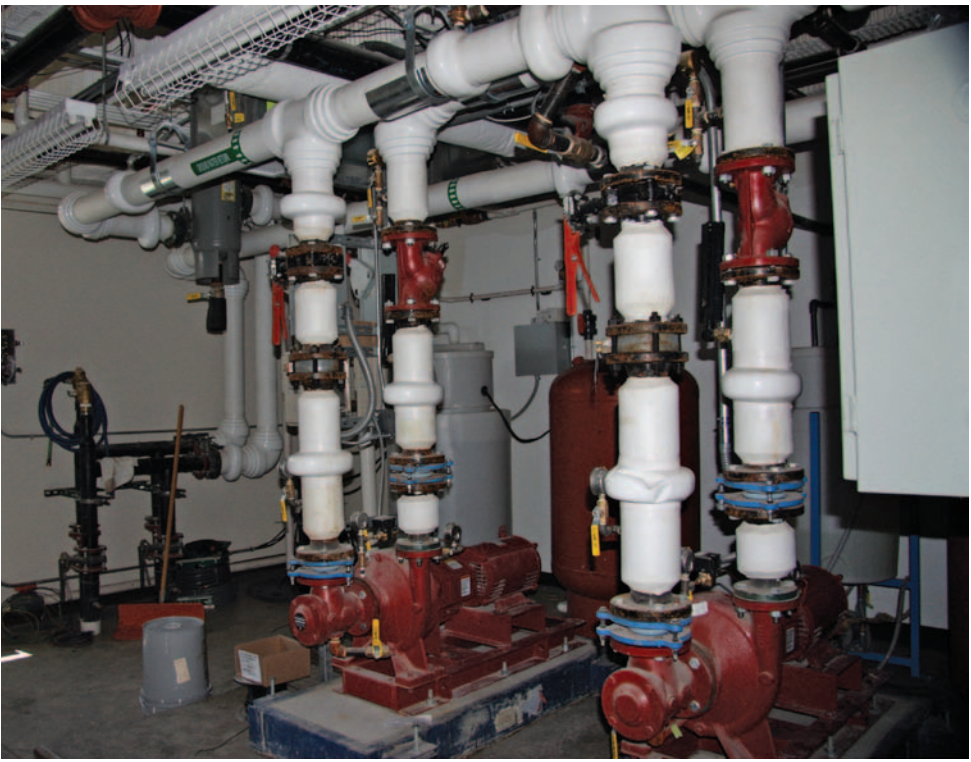
New and existing GSHP systems, like this one in Greensburg, Kansas, are a sign of resource potential in your area.
