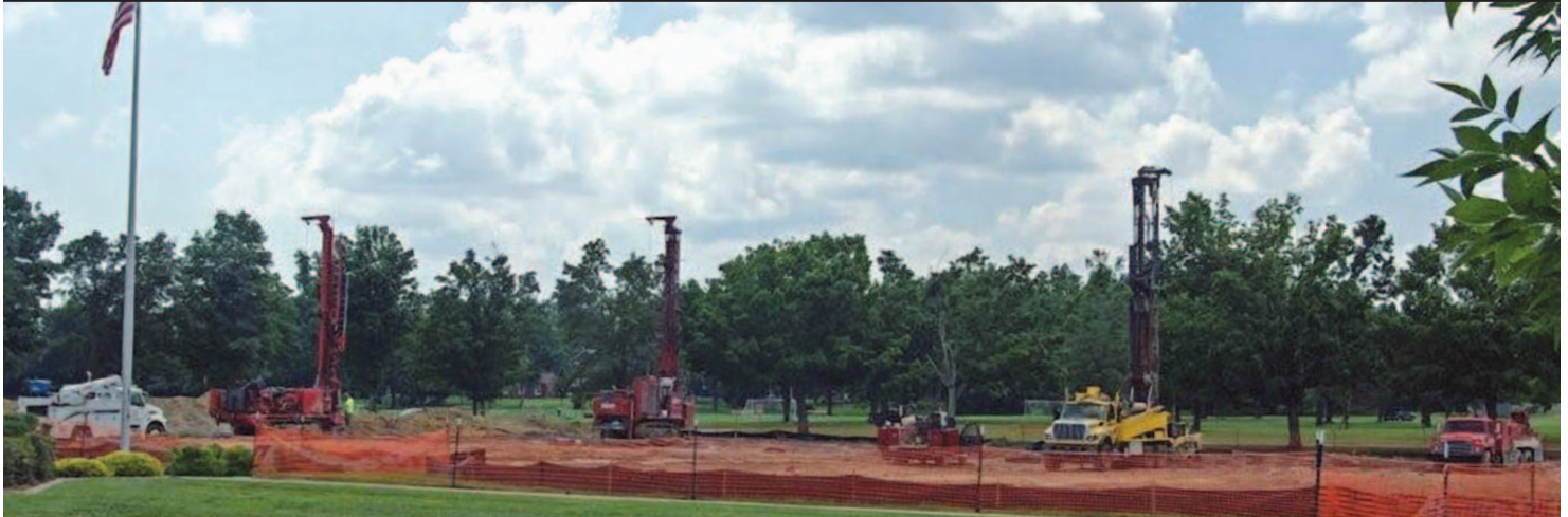
Boreholes being drilled for a ground coupled heat pump system to provide heating and cooling at the U.S. Army Fort Knox Disney Barrack, completed in 2005. Fort Knox is home to one of the largest geothermal heating and cooling systems in the world.
