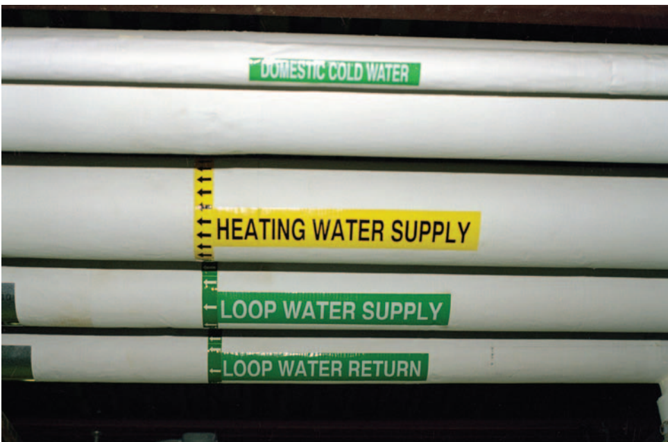
Thanks to effective geothermal policy, this elementary school in Lincoln, Nebraska, uses loop water piping as part of the school's GSHP system, shown here, to save energy and money.
