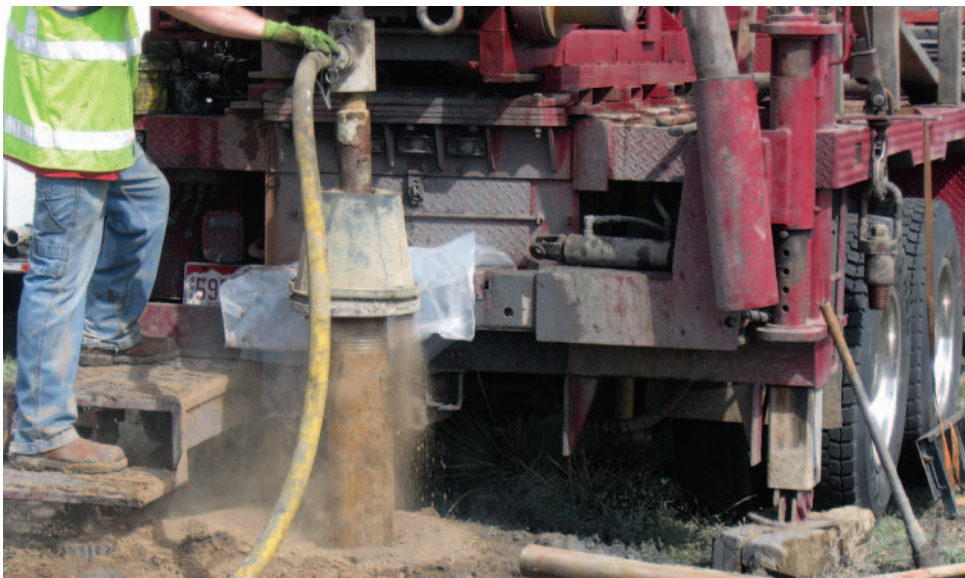
Well core drilling at the IKEA construction site in Denver, Colorado, where 130 GSHP wells, 500-foot-deep each, were dug in August 2010, showcasing how a GSHP system can be used in a commercial setting.
