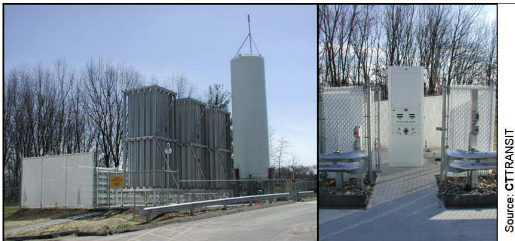
Figure D-2. Fueling facility (left) and dispenser (right) at UTC Power headquarters
