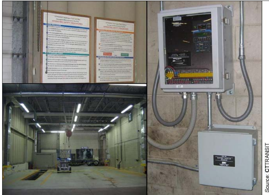
Figure D-1. CTTTRANSIT fuel cell bus maintenance bay (lower left), operating procedures (upper left), and alarm control system (right)
