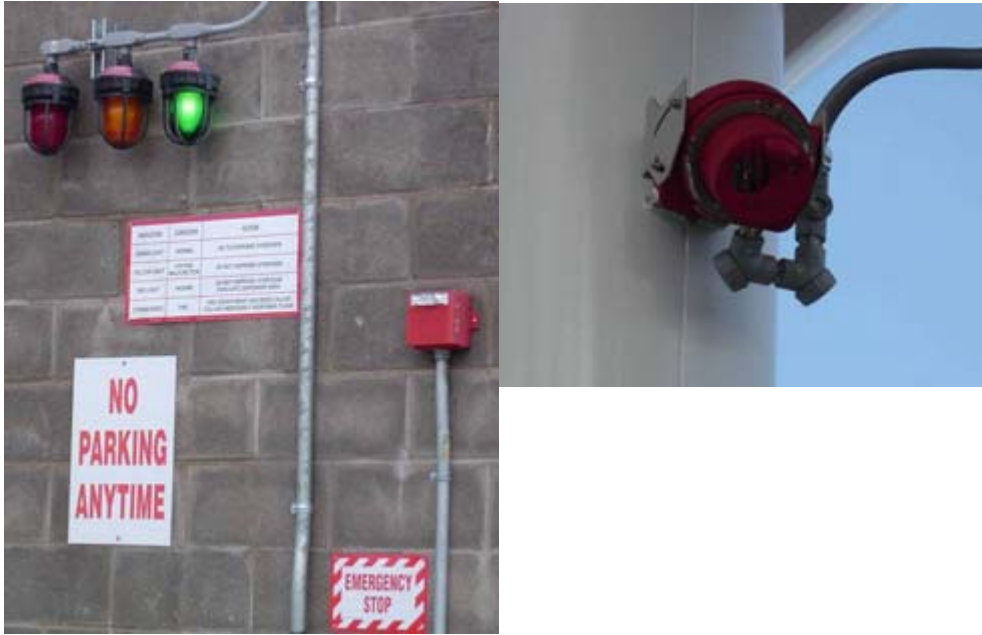
Figure 9. Condition indicator lights (left) and hydrogen flame sensor (right) at the Chevron – AC Transit Hydrogen Energy Station
