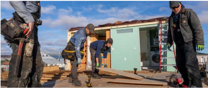
Photo by Werner Slocum, NREL 74136
