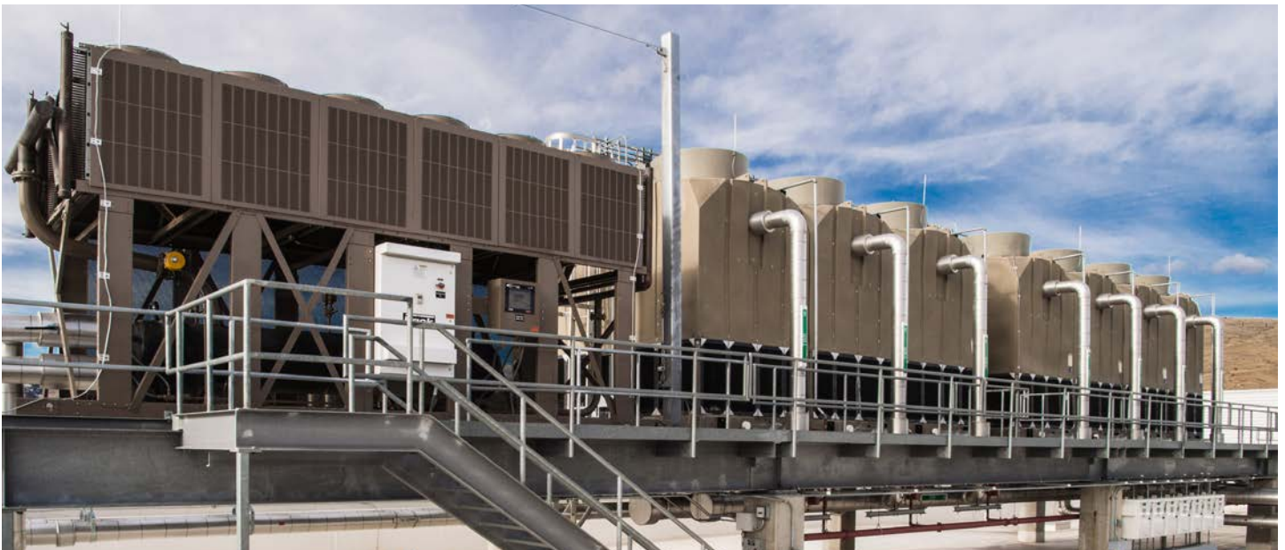
The thermosyphon cooling system sits on top of NREL's Energy Systems Integration Facility, which houses the HPC data center. The installation required only a 1-day outage to the data center. Photo by Dennis Schroeder, NREL 41999.
