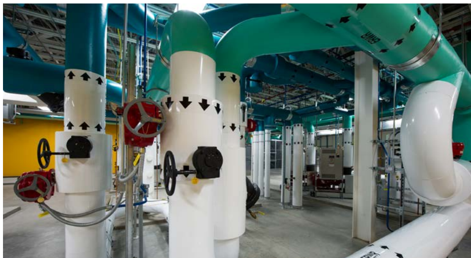
Photo by Dennis Schroeder, NREL 24645.
