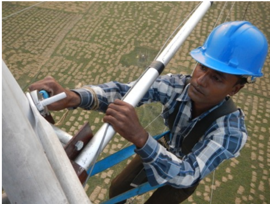
Figure 11. Local tower technician working on the tower in Sitakunda. Photo by Harness Energy.
