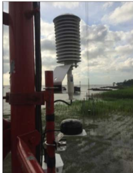
Figure 16. Temperature sensor at Chandpur. Photo by Harness Energy.
