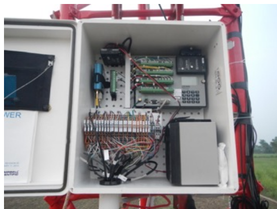
Figure 19. Enclosure with data logger. Photo by Harness Energy.
