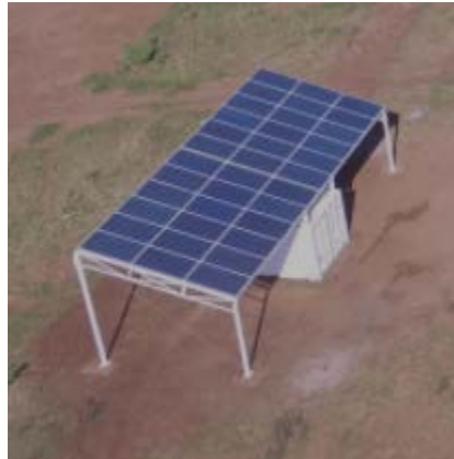
Figure 6. Standard Microgrid pilot project. Photo from Standard Microgrid.
