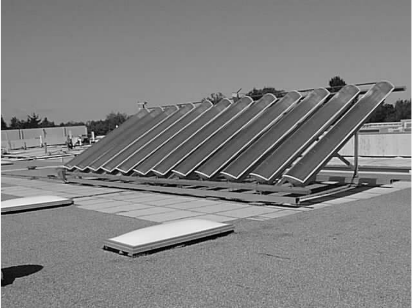
Figure 1, New PVI Powergrid on PVI Roof
