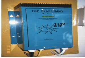
21. Beijing - Solar Roof's Inverter
