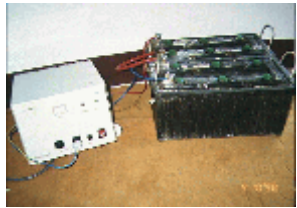
49. Hohhot - Demo House's Storage and Inverter
