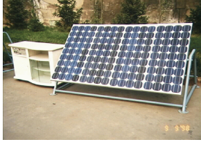
1. Xining - Distributor's Large PV Array
