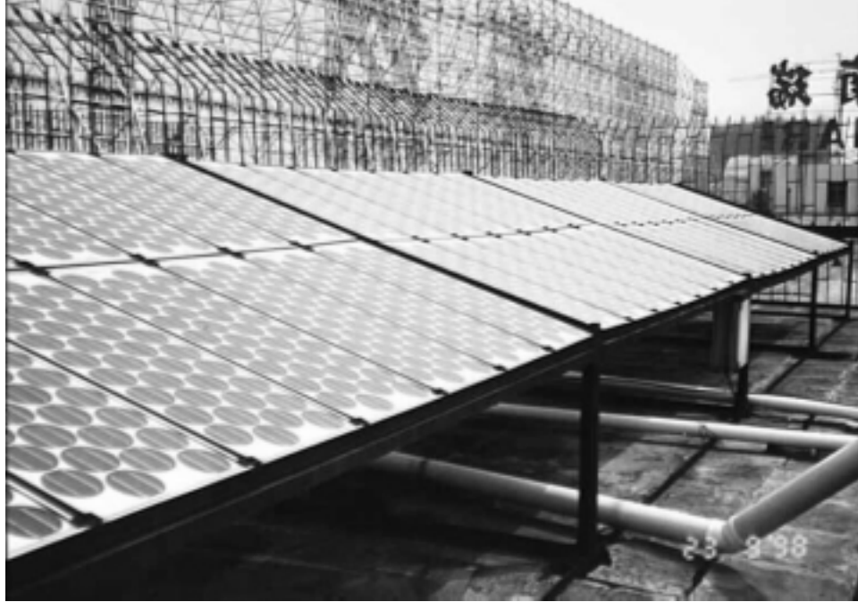
Figure 16. Shenzhen roof-mounted array
