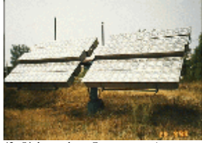
42. Qinhuangdao - Concentrator Array
