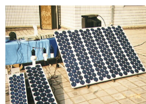
12. Lanzhou - Rooftop Demo
