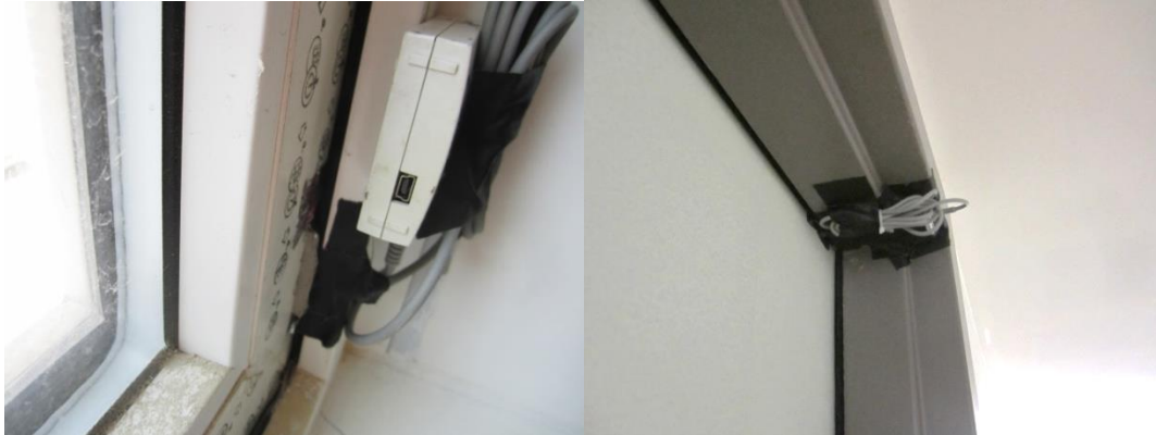
Figure 34. Contact closure data loggers to monitor window opening (left); door opening (right)
