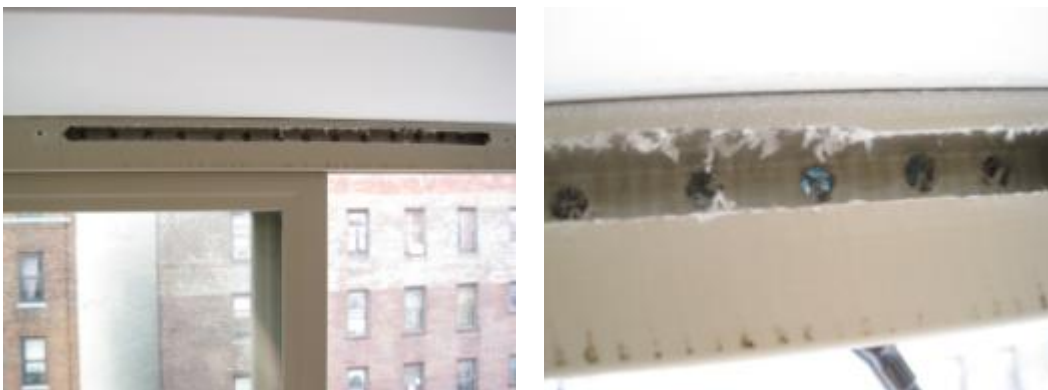
Figure 12. Cut for trickle vent in window frame (left), trickle vent removed; close-up of the opening (right)
