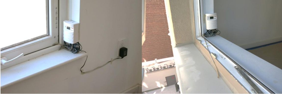
Figure 7. Placement of window data loggers for pressure measurement (shown without exterior shield)
