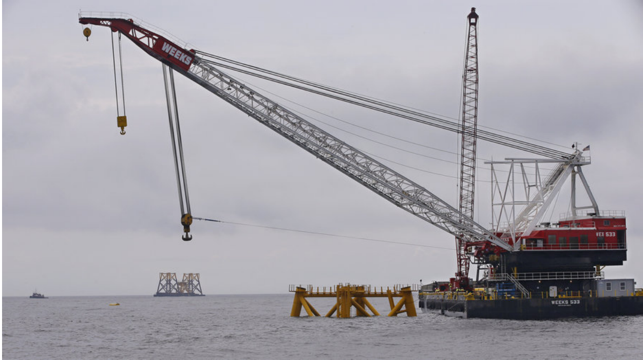
Figure 9. The 30-megawatt Block Island Wind Farm under construction. Photo courtesy of Deepwater Wind
