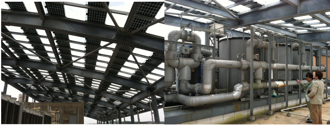
Figure 13. Itoman City Hall building photovoltaic system (left) and cold brine storage (right)
