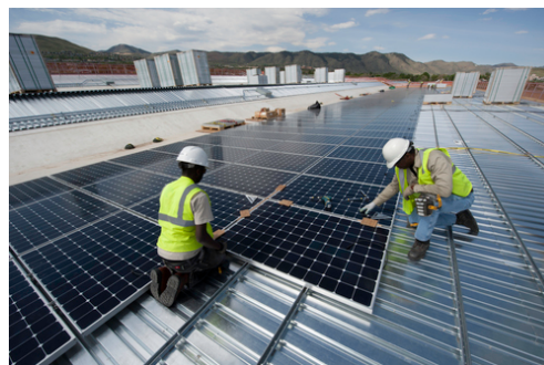
Figure 12. Example of rooftop photovoltaic system
