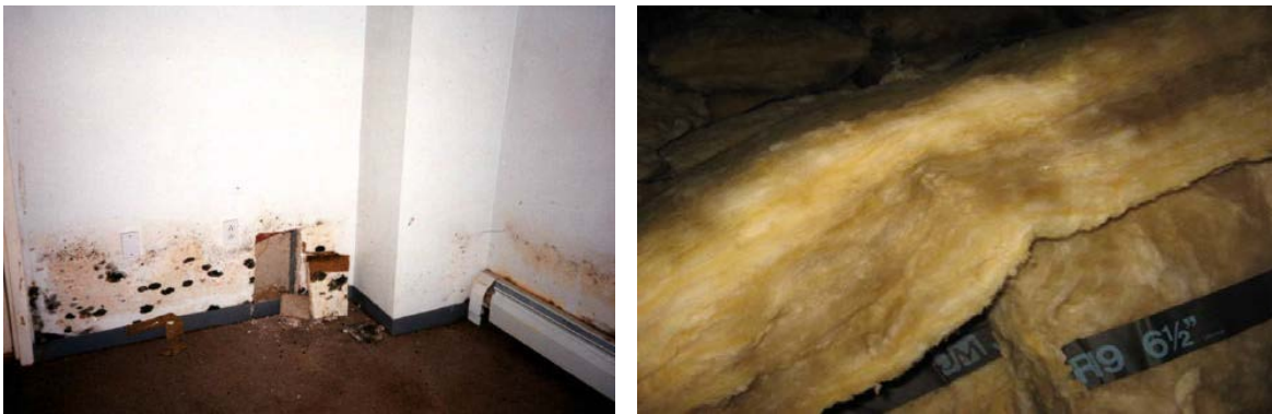
Figure 7. Signs of poor air sealing and insulation performance
