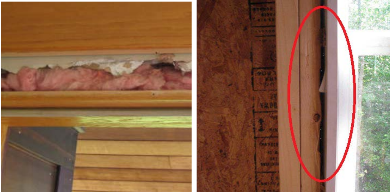
Figure 8. Poor air sealing around windows (ENERGY STAR 2011c) (Left photo courtesy Efficiency Vermont; right photo courtesy U.S. Department of Energy)
