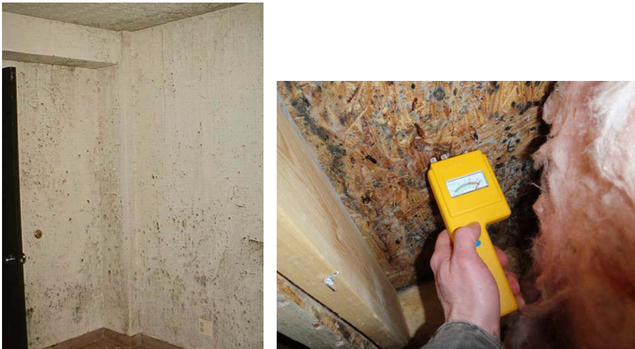
Figure 6. Mold growth on the inside surface of exterior walls (left) and inside the wall cavity (right). Both conditions are likely caused by an improperly air sealed and insulated wood-framed wall assembly.
