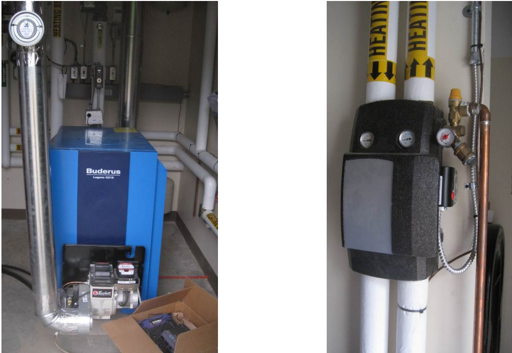
Figure 12. Replacement boiler with microprocessor controls (left); associated water flow control (right)
