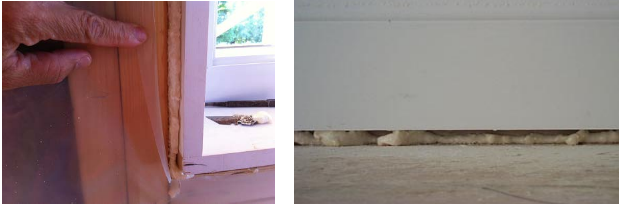
Figure 9. (Left) Good air sealing around windows and (right) between drywall and subfloor (Photos courtesy Efficiency Vermont)
