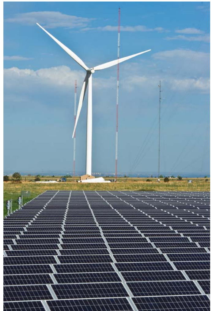
Photo by Dennis Schroeder, NREL/PIX 20689
