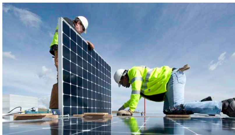
Photo by Dennis Schroeder, NREL/PIX 21499
