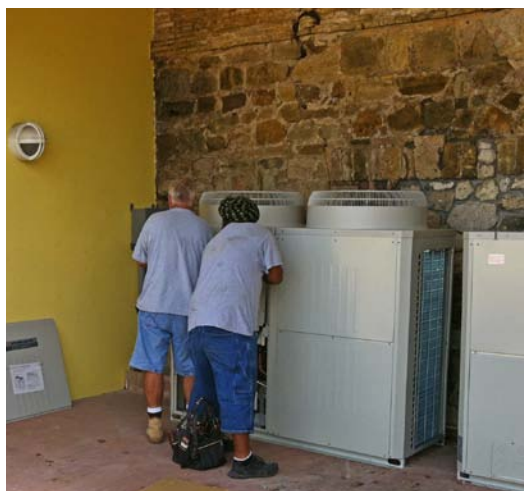
Contractors replaced 64 tons of inefficient heating, ventilation, and air-conditioning (HVAC) equipment with 48 tons of highly efficient variable-refrigerant-airflow system that will cut the historic Bjerget House buildings' energy use by an estimated 37%. Photo from Quality Electric Supply Inc., NREL/PIX 20813
