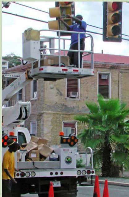
DPW workers install energy-efficient LED traffic lights at a Charlotte Amalie intersection, St. Thomas. Photo from Don Buchanan, VI Energy Office, NREL/PIX 20814
