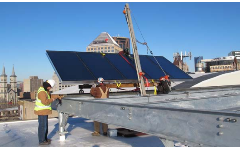
Local installers inspect PV panels that are part of the District Energy Saint Paul Solar Thermal project. Photo from District Energy, NREL/PIX 18697
