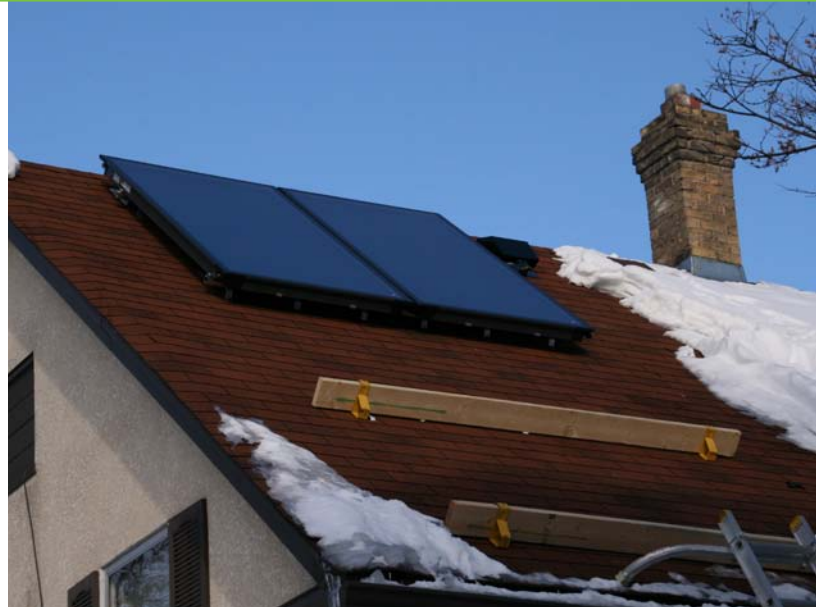
Residential areas also are adopting solar power. Here, a rooftop installation is displayed on a home. Photo from Applied Energy Innovations, NREL/PIX 18699
