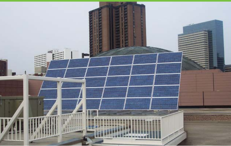
A rooftop solar array system is displayed on a Minneapolis business. Photo from Meet Minneapolis, NREL/PIX 18698
