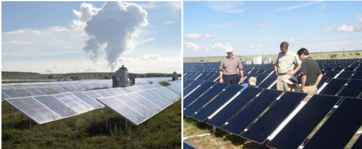
Figure 1 PV sub-arrays at Tucson Electric Power in Springerville, AZ, made with 300 W (left) and 50 W (right) modules.
