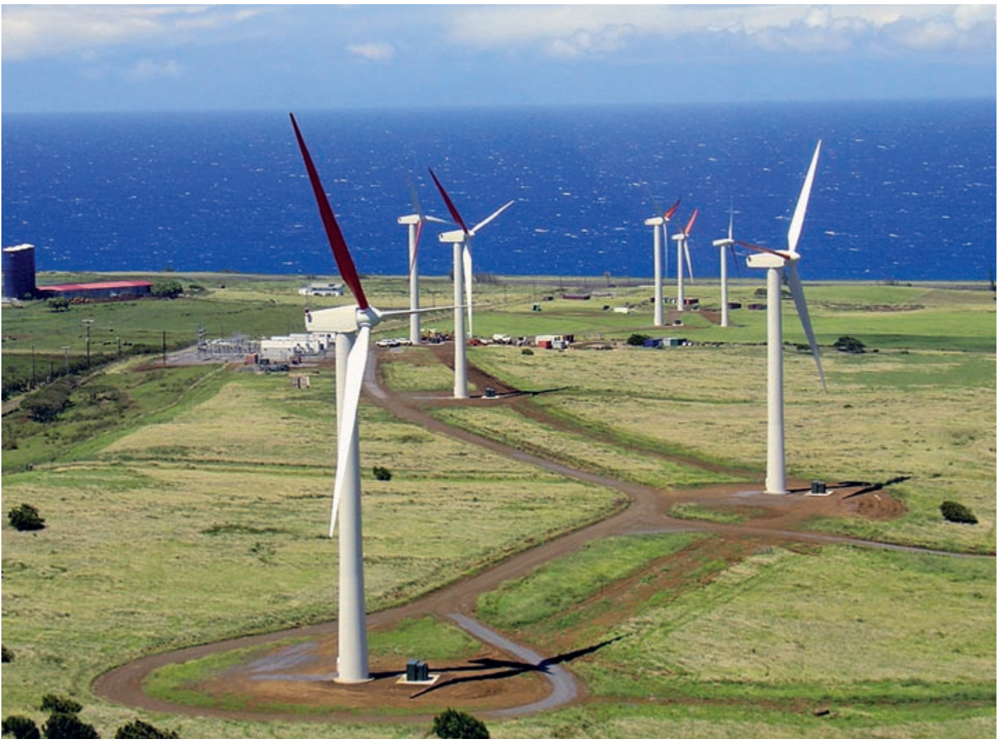
The 10.5-MW Hawi Renewable project at Upolu Point on the Big Island utilizes 16 Vestas V-47 660-kW turbines. Photo credit: Hawaiian Electric Light Company (HELCO)/PIX14697
