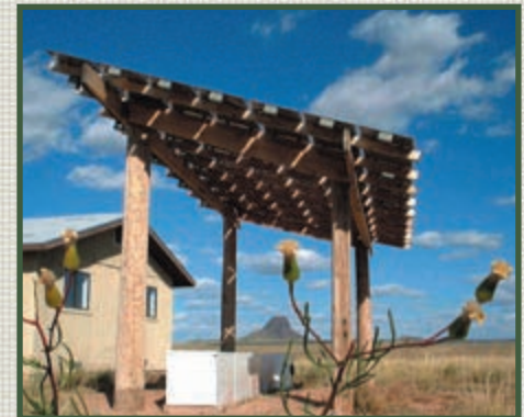
Solar electric array on Navajo home
