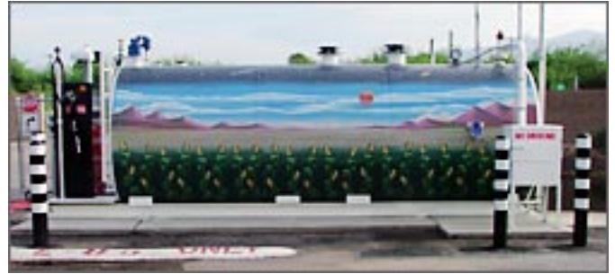
The University of Arizona installed this 4,000-gallon above-ground ethanol tank.
