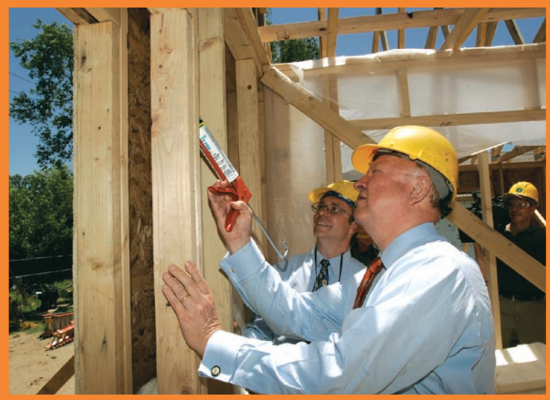
Secretary of Energy, Samuel Bodman, gives a hand in the construction of the National Renewable Energy Laboratory 2005 Habitat for Humanity house in Wheatridge, Colorado. This highly efficient, solar-powered house will generate as much energy as it consumes. Credits: NREL/PIX14017 (above); NREL/PIX11977 (upper right)
