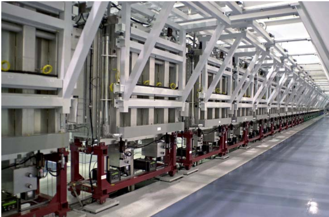
Fig. 2. Side view of the United Solar 30 MW/yr a Si processor.
