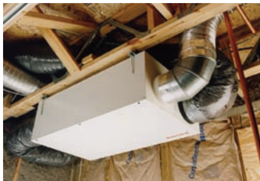
An energy recovery ventilator ensures good indoor air quality.
