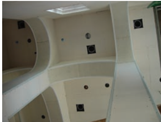
Dramatic 20-foot ceilings that have been carefully ducted show the marriage of pre-1940 style with modern efficiency.
