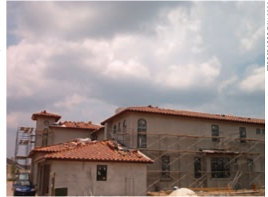
The roof is made of red clay tile that is characteristic of traditional Florida homes.
