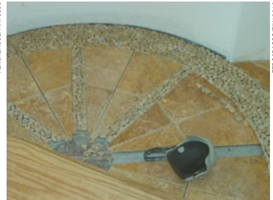
The home reflects care for detail, such as the pattern in these floor tiles.
