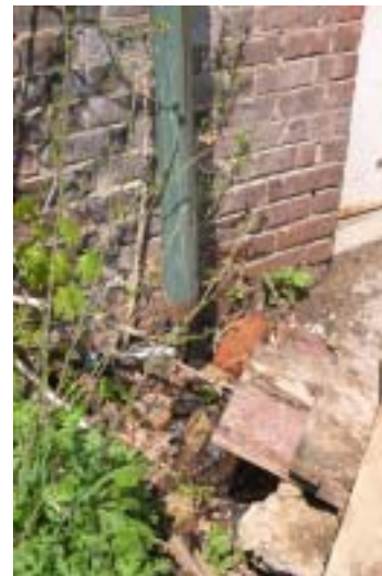
Fig. 14: Damaged downspouts are a source of water penetration through the foundation wall.
