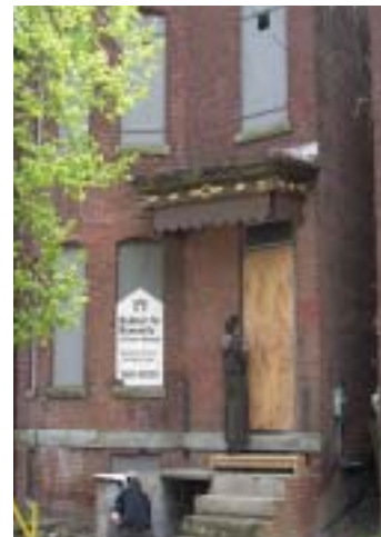
Fig. 13: Rebuilding the porch prevents further water damage to the foundation of this home.
