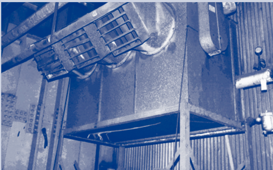
Steam Heater for the Tin Mill (Project 6)
