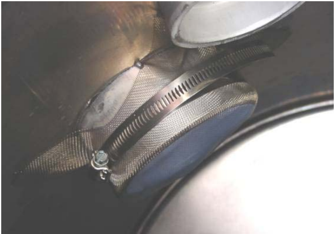
Figure B-2. Tank No. 1 – Internal View of Screen-Type Flame Arrester.
