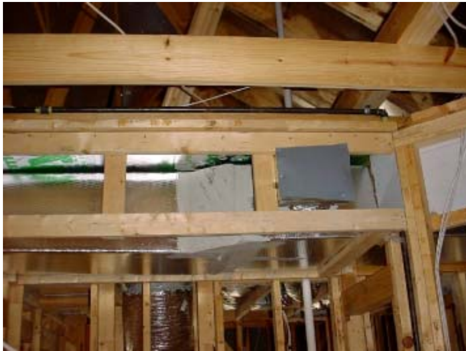
Figure 9. The final duct installation incorporated a horizontal duct board trunk in the bulkhead with flex duct runs perpendicular to this main trunk.
