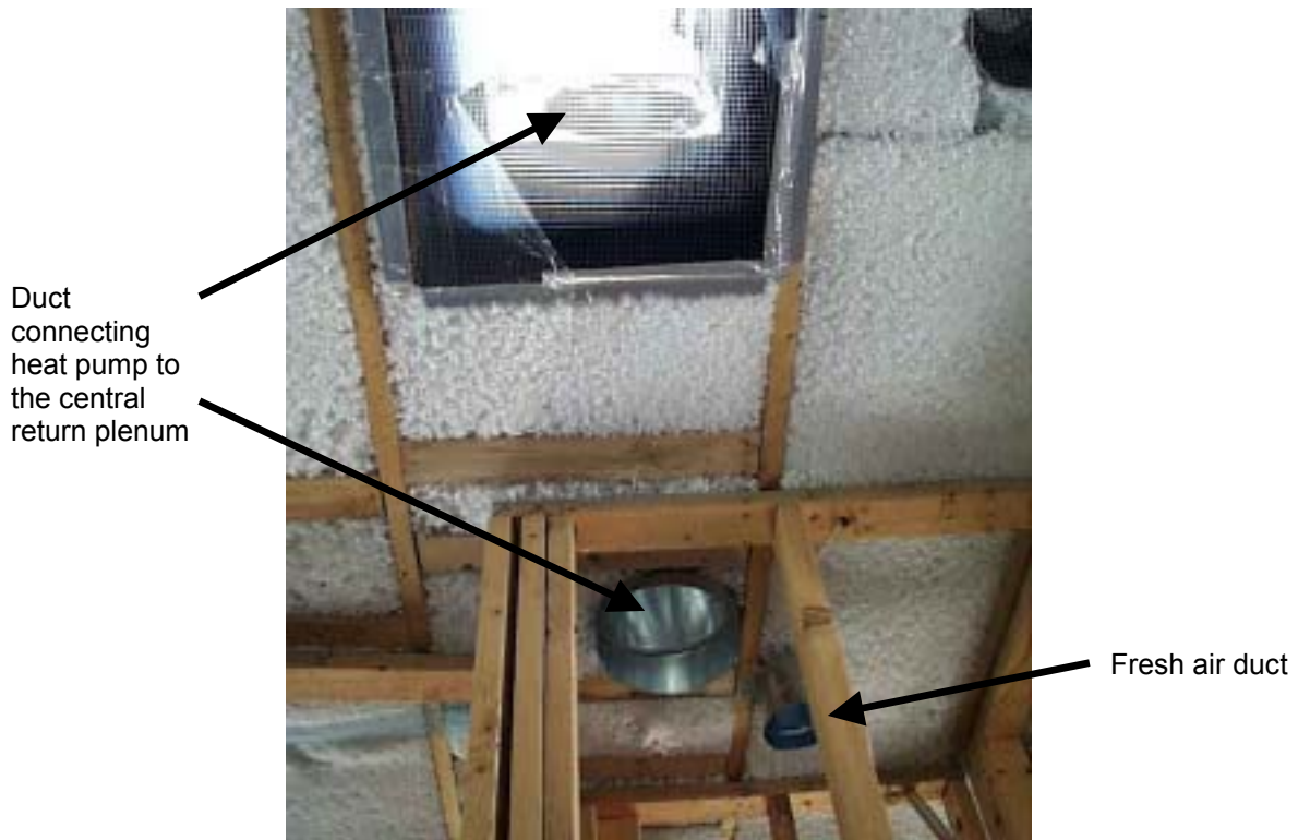
Figure 25. A 5-in. fresh-air duct penetrates the top of the closet where the heat-pump water heater will be installed. This outdoor air will be mixed with house air pulled from the closet (connected to the hallway with a louvered door). The cooled air leaving the heat-pump water heater is connected to the central return plenum in the attic.
