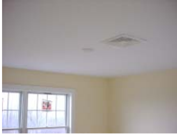
Figure 15. The four-way throw supply diffusers are 6 to 10 ft away from the perimeter and distribute air evenly throughout each of the smaller bedrooms.
