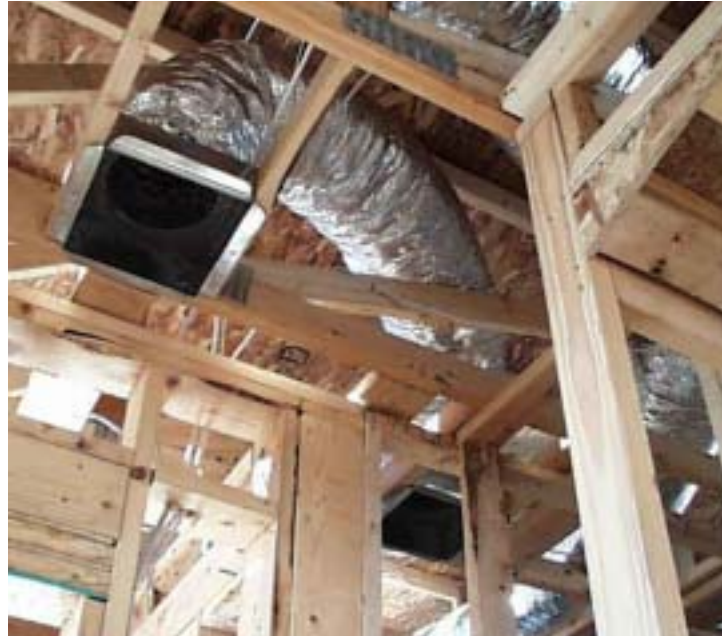
Figure 23. Jump ducts are successfully used to transfer return air from the bedrooms to the central hallway space.
