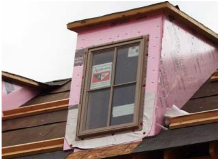
Figure 30. Dupont® FlexWrap™ was used to flash the windows. The sill was flashed before the window was installed.
