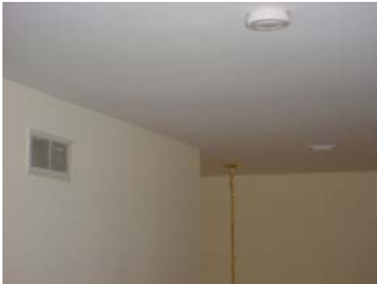
Figure 17. The ventilation ceiling register (on right) is about 9 ft away from the second-floor central return.
