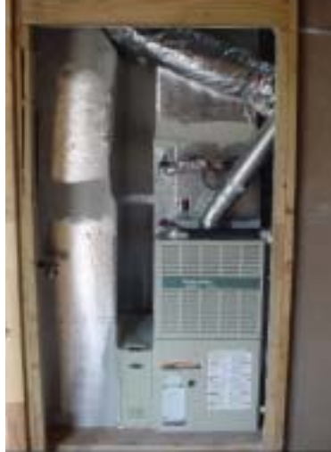
Figure 10. A fresh-air intake duct with a constant airflow regulator runs from the outside to the return plenum. The furnace operates continuously on low speed to provide whole-house ventilation.
