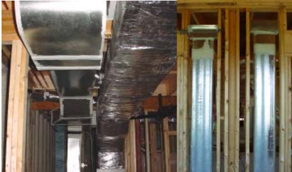
Figure 14. On the left is an example of the careful mastic sealing done on a return trunk line that runs beside a sealed and insulated supply trunk. On the right are two return branches that terminate in the high wall on the first floor with mastic sealant at joints and foil-faced tape on the longitudinal seams of the sheet metal oval ducts.
