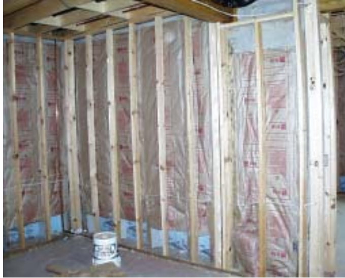
Figure 13. R-19 batt insulation filled the cavities of the Superior Wall foundation (insulation gaps and band joists were filled in later). Because the drywall finish in the basement was extremely important, a stand-alone frame wall was set in front of the foundation.
