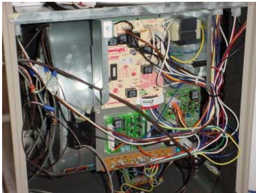
Figure 3. Analyzing the fan and furnace control system was a key part of evaluating the performance of the home. The control settings inside each unit were evaluated to ensure that air distribution performance would meet design goals.
