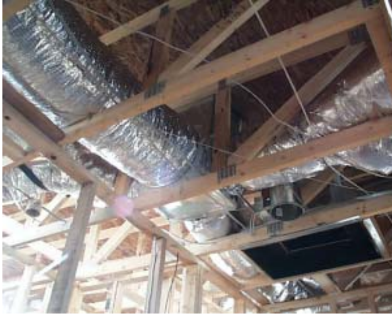
Figure 22. Flex duct runs branch out from the central supply plenum to the various rooms in the house. The central return grille and plenum are located directly below the air-handling unit on the roof to minimize duct length and leakage points.
