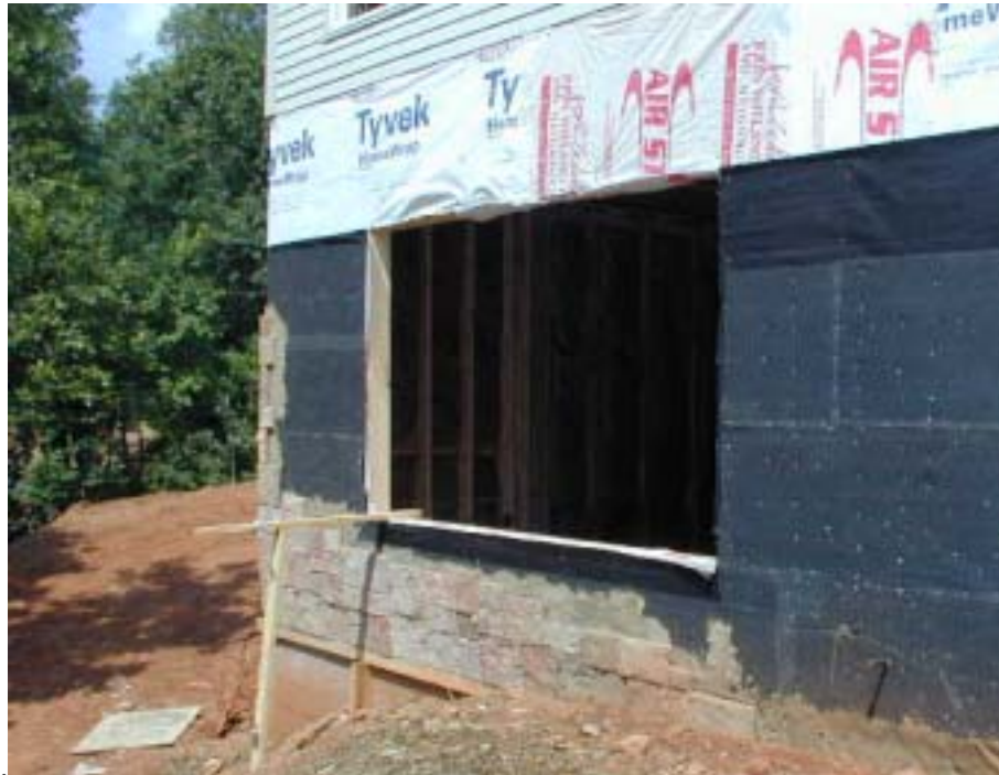
Figure 5. Building felt was used to provide greater wall moisture protection behind the cultured stone. Membrane flashing was used to cover the sill rough opening. The top window flange was slipped under the housewrap (above), after the window was installed with its flanges back-caulked (except for the sill flange).
