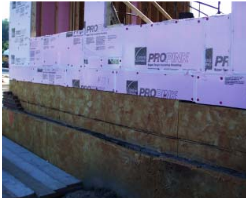
Figure 29. The foundation walls were insulated above and below grade with semirigid fiberglass board. XPS insulation board was used on all above-grade walls and taped to improve airtightness and create a drainage plane.
