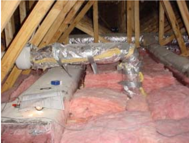
Figure 16. The portion of the ventilation system from fan to the diffuser is shown. It was insulated to prevent condensation. Ductwork in the attic is insulated with R-6. To ensure full and even attic insulation coverage, ductwork was raised above the drywall (at left). The ventilation register is at the edge of the two-story foyer space.
