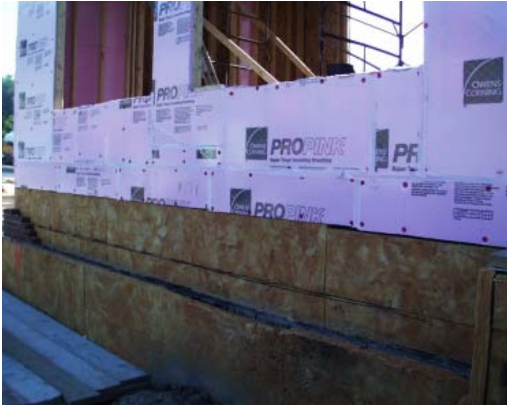
Figure 27. The foundation walls were insulated on the exterior below grade and above grade behind the brick veneer. The above-grade walls had ½-in. OSB at corners covered with ½-in. XPS insulation board, with 1-in. XPS insulation board on the rest of the wall.
