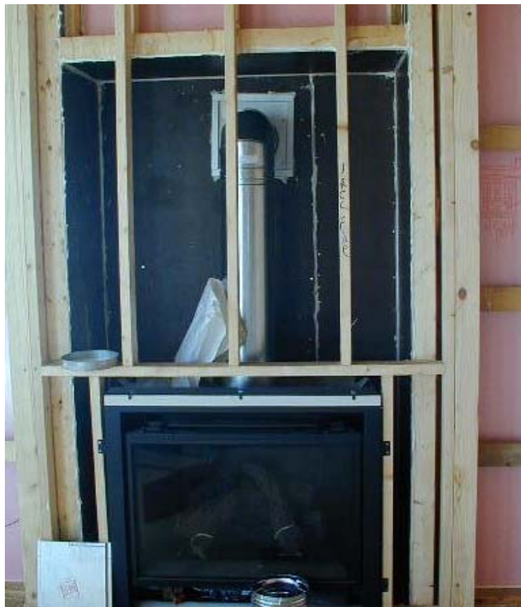
Figure 28. Draftstopping was installed behind tubs, shower surrounds, fireplaces, and duct chases. These wall cavities were preinsulated, and the draftstopping was caulked to the framing members on all edges.
