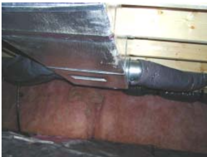
Figure 7. The builder constructed an unvented crawlspace with insulated walls and a source for conditioned air.
