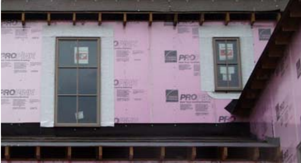
Figure 31. After the window was installed, FlexWrap™ was installed on the jambs, then across the window head.
