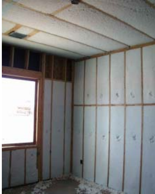
Figure 21. Blown-in-place fiberglass insulation is installed in the exterior walls and ceiling before drywall is installed
