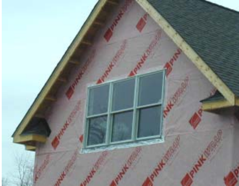
Figure 18. Based on discussions at the time of the benchmarking visit, the builder has now instituted a window and door flashing strategy. The builder was instructed in the correct sequence for placing the membrane flashing as well as the best time to install the window and its integration with the plastic housewrap. The application in this photo occurred several months before pilot home construction began; although the sill flashing was installed incorrectly at that time, it is a step in the right direction and a major advancement for the builder.
