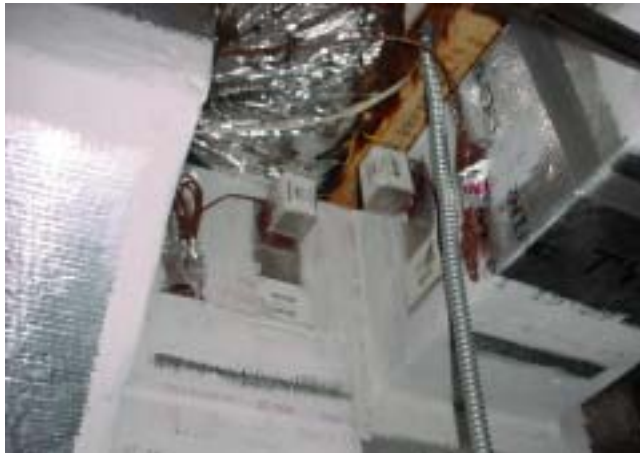
Figure 2. The home has five zone dampers; two can be seen on supply ductwork coming from one of the two air handlers.
