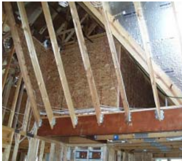
Figure 4. The child's loft is located in attic space behind the vaulted roof rafters. The OSB sheathing was installed on its outward-facing walls to separate the loft space from the attic, thereby improving building airtightness and thermal performance.
