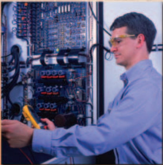
A researcher monitors the control panel for a simulated utility grid at NREL's Distributed Energy Resources Test Facility. Using the control panel, researchers can adjust voltage, frequencies, loads, and a variety of other parameters to determine how the network may work under different conditions.
