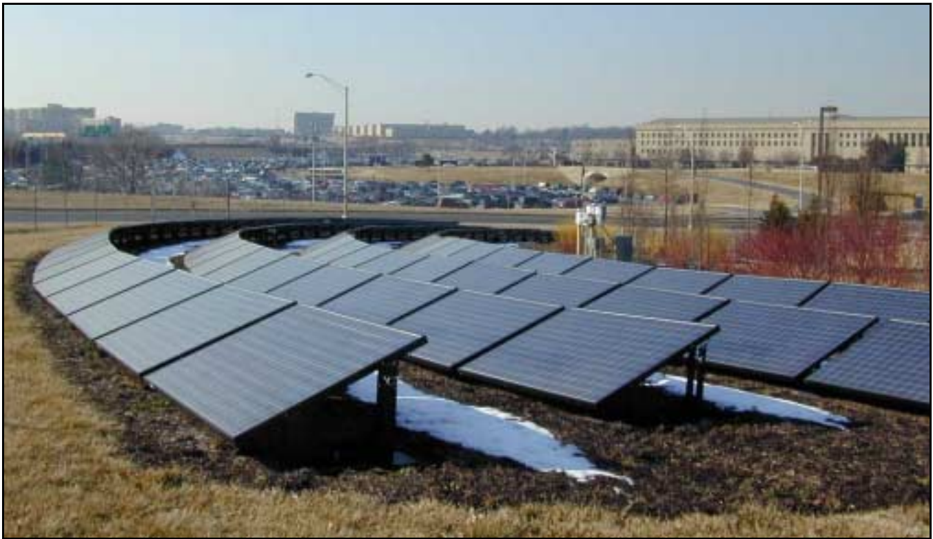
Figure 3. View of the Pentagon's ground-mounted 30-kW PV system showing 4 arcs of PV modules. (Photo: P. Plympton)
