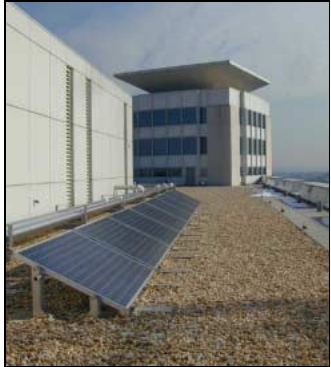
Figure 4. View of roof-mounted FERC PV system. (Photo: P. Plympton)
