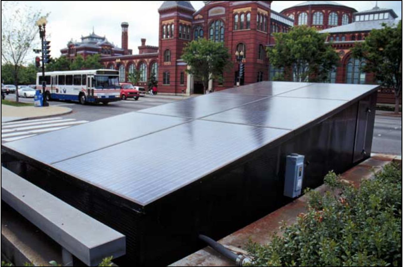
Figure 1. View of the Earth Day Park PV system. In the background across the street is the Smithsonian's Arts and Industries Building. (Photo: B. Stafford)
