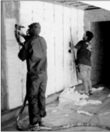
Figure 13. Spray foam insulation can be used between a garage and the home to make an air barrier that isolates the home from the carbon monoxide produced in a garage.
