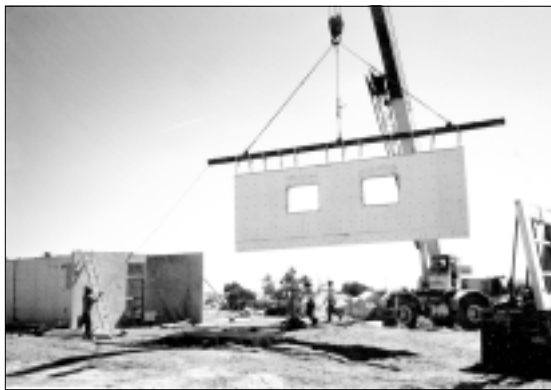
Figure 25. A concrete panel that was poured in a factory off site is lifted into place by crane.
