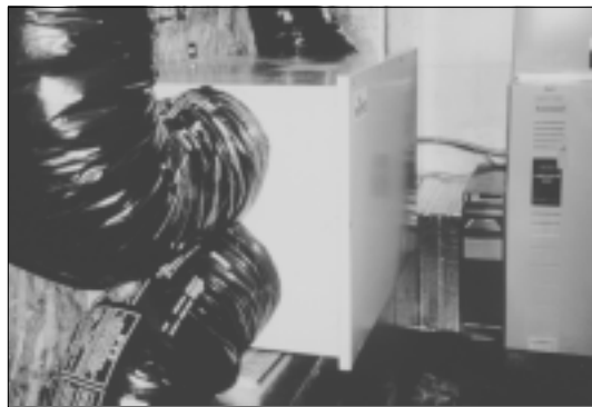
Figure 12. A heat recovery ventilator brings fresh air into a house without sacrificing energy efficiency.
