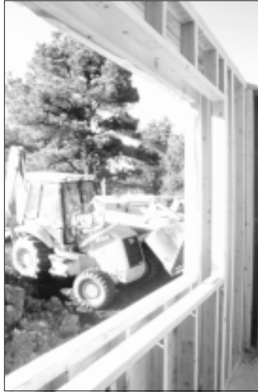
Figure 24. A double wall system was used to create an R-38, fiberglass batt-insulation wall.
