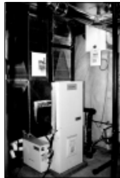
Figure 42. Interior geothermal equipment.
