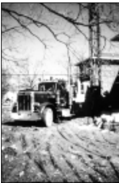
Figure 40. A vertical bore hole is dug for a geothermal loop by using well-drilling equipment.
