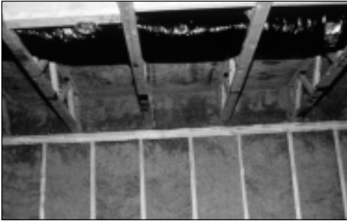
Figure 35. Ductwork in unconditioned space should be well-insulated.
