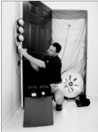
Figure 9. Blower door tests are required for most home energy ratings and usually cost $200 or more.
