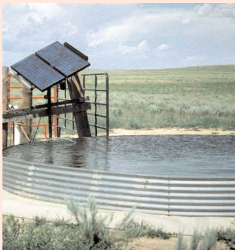
This portable PV system pumps 1.75 gallons per minute from a 60-foot well to fill a remote stock tank.
