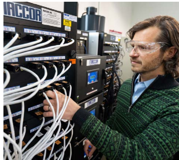
NREL's BTMS research evaluates how next-generation battery designs can meet the unique demands of stationary storage.
