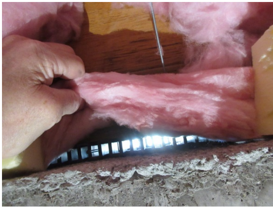
Vented Crawl is not sealed
