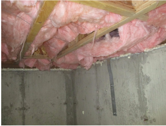
Poorly done insulation in the crawl space ceiling
