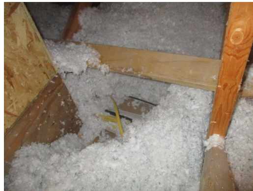
Missing attic insulation garage access
