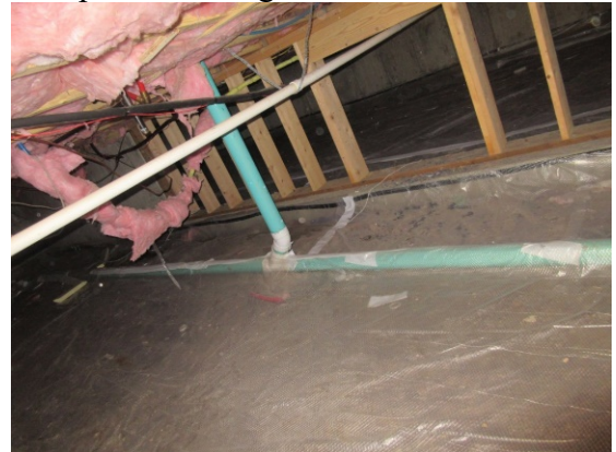
Poorly insulated pipes, and radon pipe
