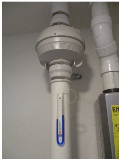
Properly connected radon fan.
