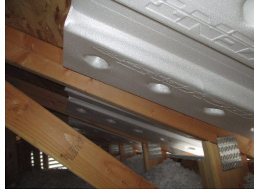
Soffit baffels – additional insulation can be added
