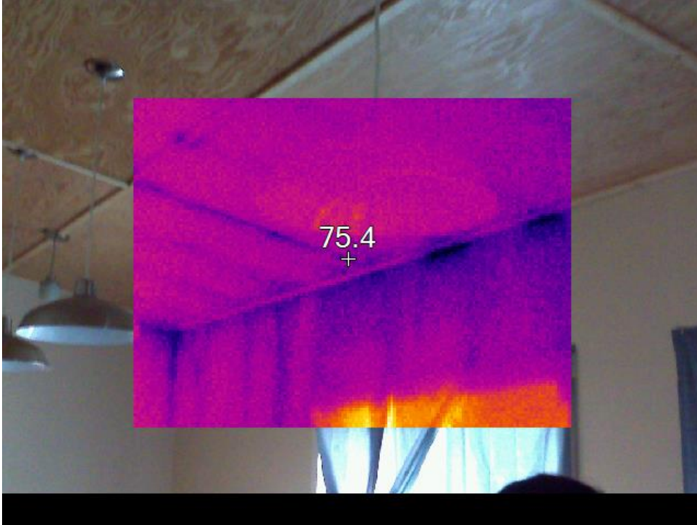
Air leakage from the attic above the kitchen family room area.
