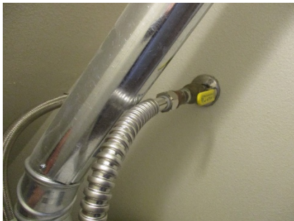
Water Supply Line resting against flue
