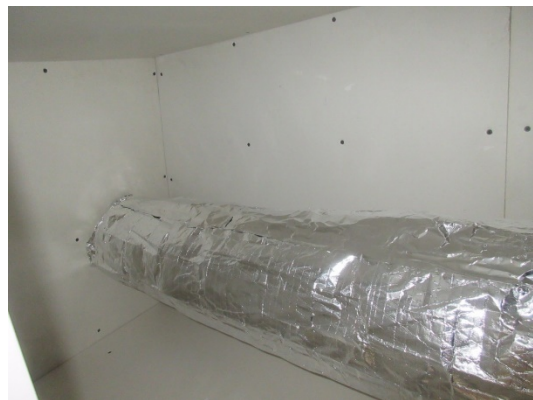
HVAC closet is not air sealed
