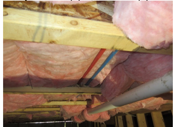
These water line are exposed to freezing temperatures
