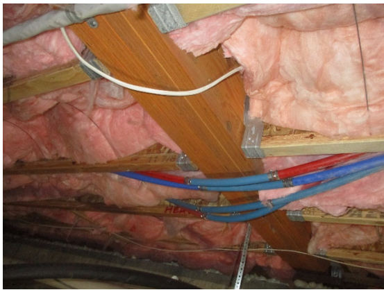
Exposed water lines in a vented crawl space
