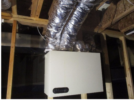
HRV Unit in crawl space
