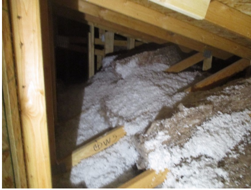
Poorly aligned batts
