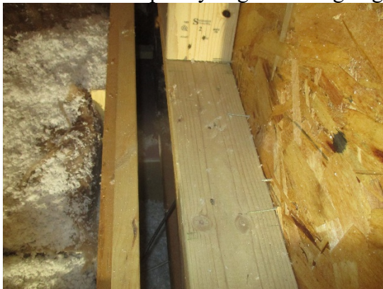
Air gap in the garage attic area
