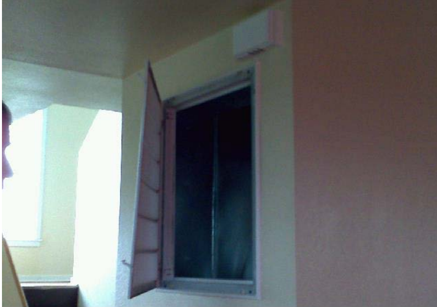
Return air duct in the home.
