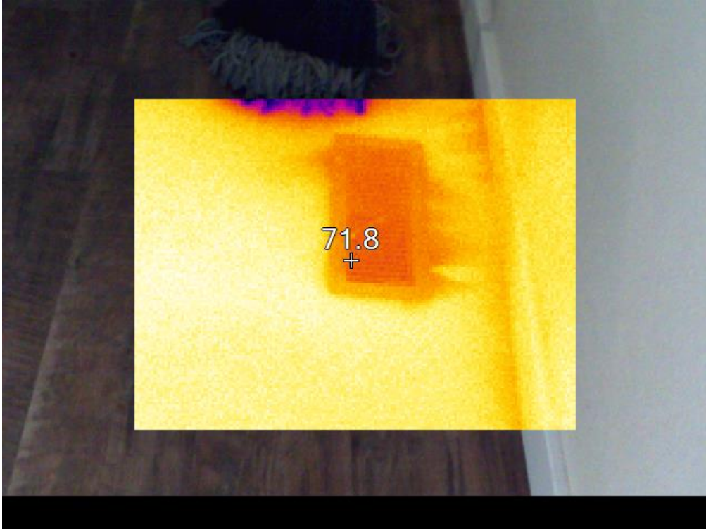
The wispy red in the image represents either rim joist leakage around the duct boot or duct leakage.
