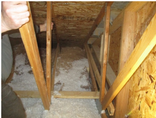
Attic Insulation poorly aligned batt/ garage access
