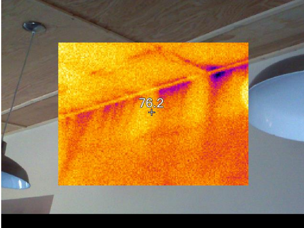
Red streaking represents air leakage.
