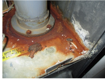
Corrosion on furnace
