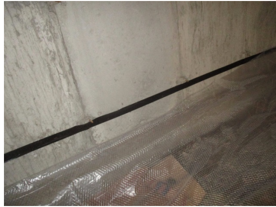
Crawl space liner is not attached to the wall
