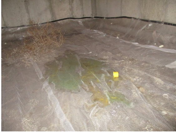
Standing water in the crawl space
