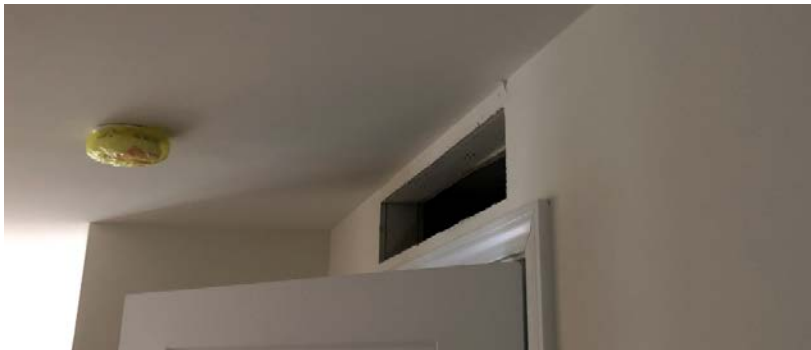
Transfer grille for AHU return air.
