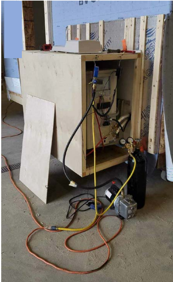
Heat pump compressor install. Gable end install so it can travel down the road.
