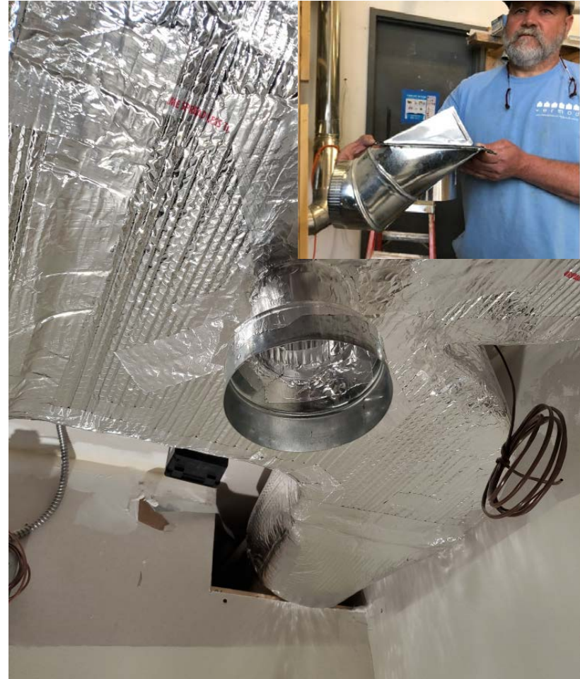
Injection port for fresh air via ERV.
