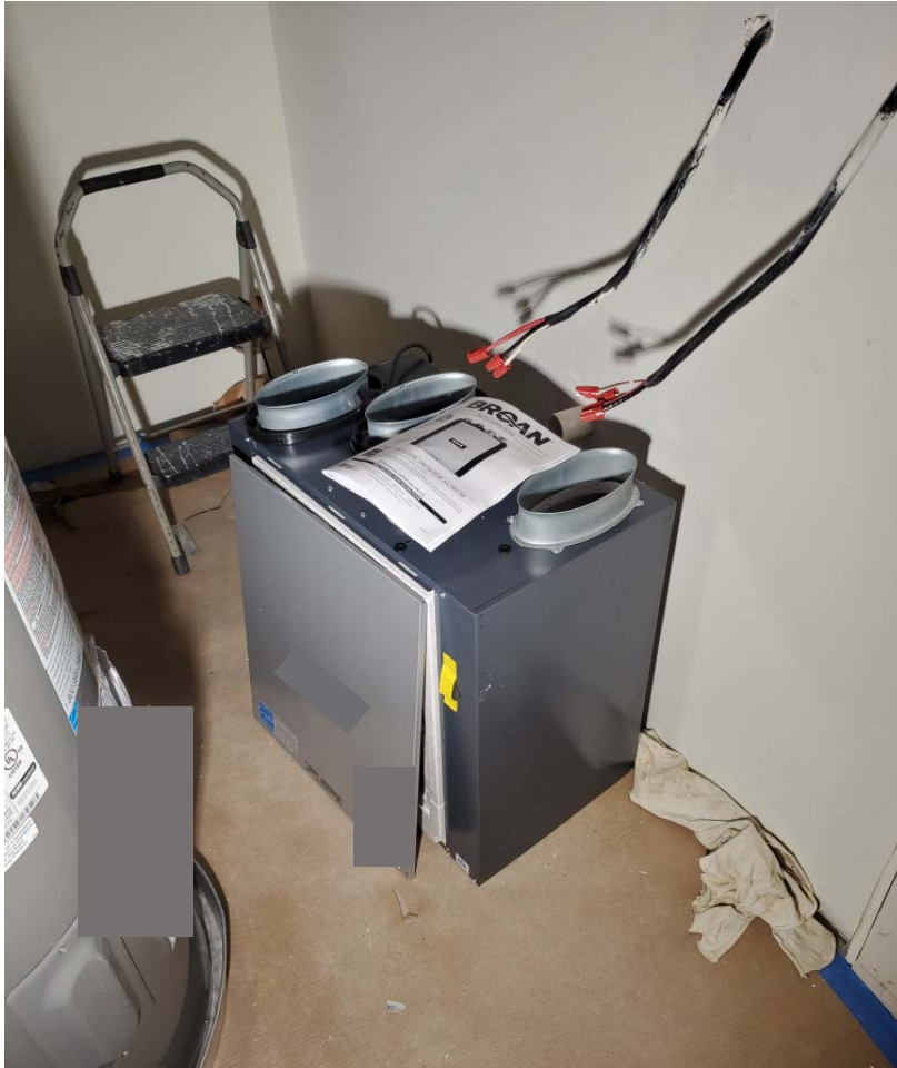
Ensuring proper space for install and future service.
