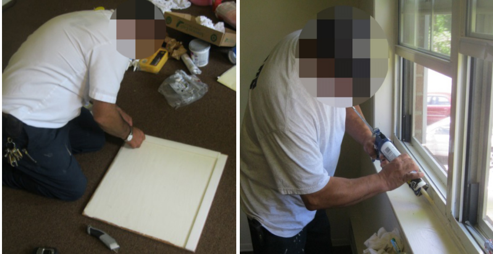
Figure 4. Installing gasket on attic hatch (left); caulking gap around window (right) at IHA
