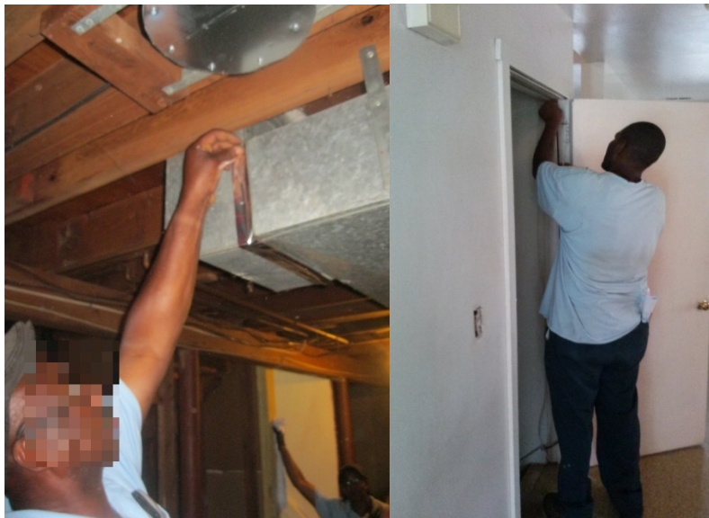
Figure 17. Sealing ductwork with Underwriters Laboratories-181 tape (left); installing weather stripping on door to unconditioned basement (right) at NHA
