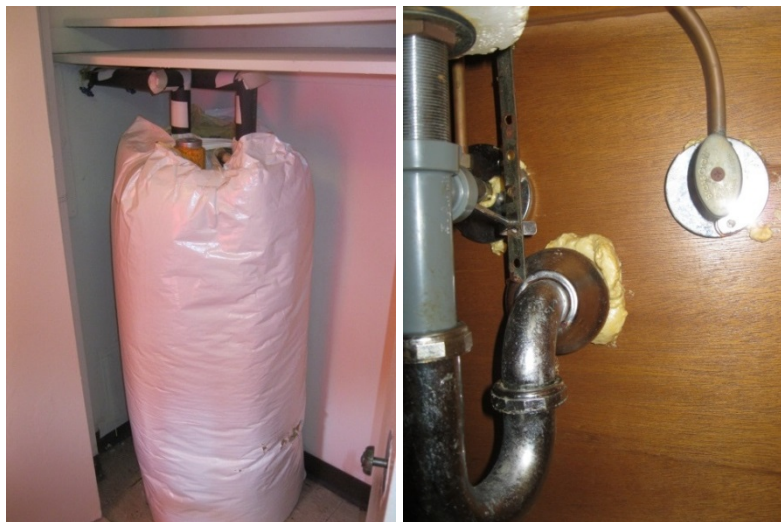
Figure 3. Electric storage water tank with insulation wrap (left); foamed plumbing penetrations (right) at IHA
