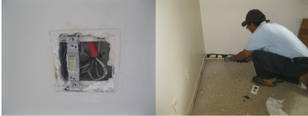
Figure 16. Newly caulked electrical outlet (left); caulking around base molding (right) at NHA
