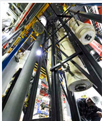
An NREL engineer inspects the newly installed re-circulating reformer in the thermochemical conversion pilot plant. Photo by Dennis Schroeder, NREL 25486
