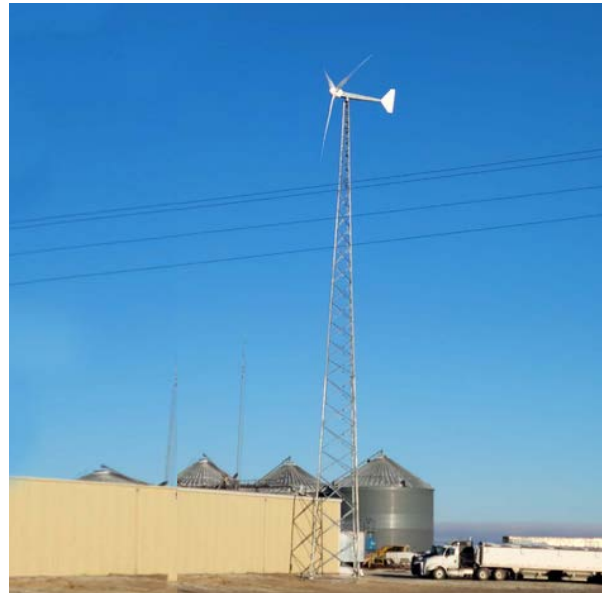
A Bergey Excel 15 turbine on a 100-foot self-supporting lattice tower at a rural business in Juniata, Nebraska. Photo from Mike Bergey, Bergey Windpower
