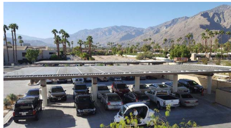
80-kW parking canopy solar system at Agua Caliente reduces annual Tribal office electricity cost from $22,000 to $200.
