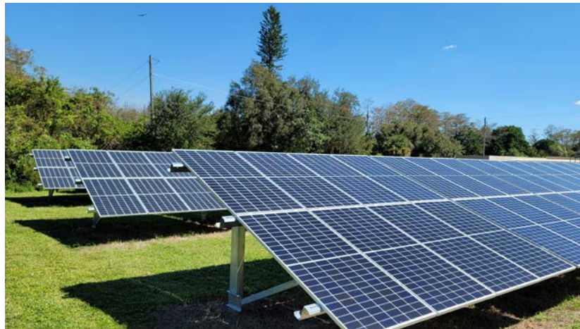
Seminole Tribe of Florida's ground-mounted solar array
