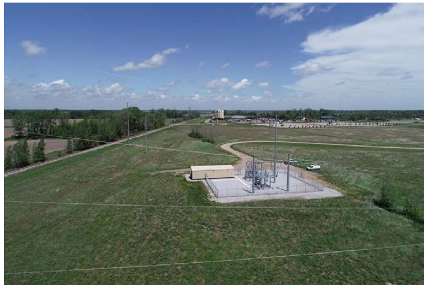
Saginaw Chippewa Indian Tribe of Michigan's substation supporting Tribal utility operations
