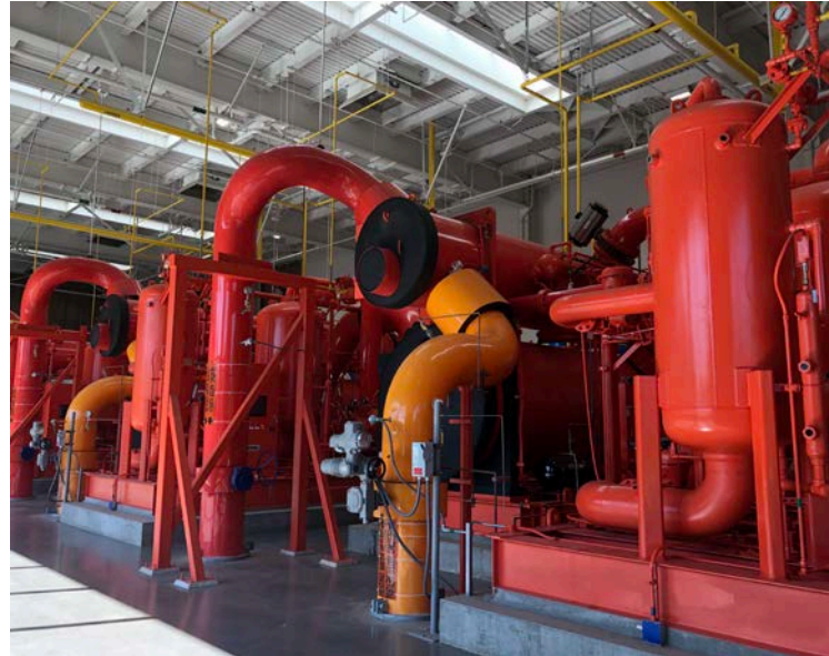
Figure. Pumps for district heating system
