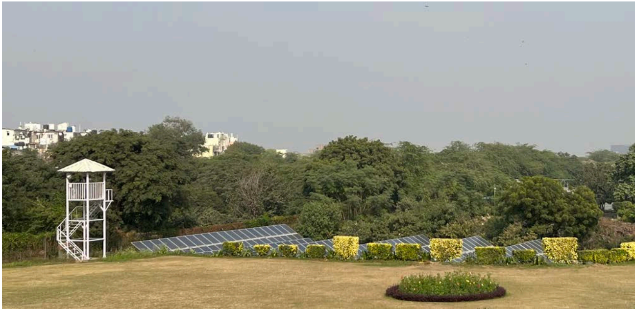
Figure. Solar power plant in India
