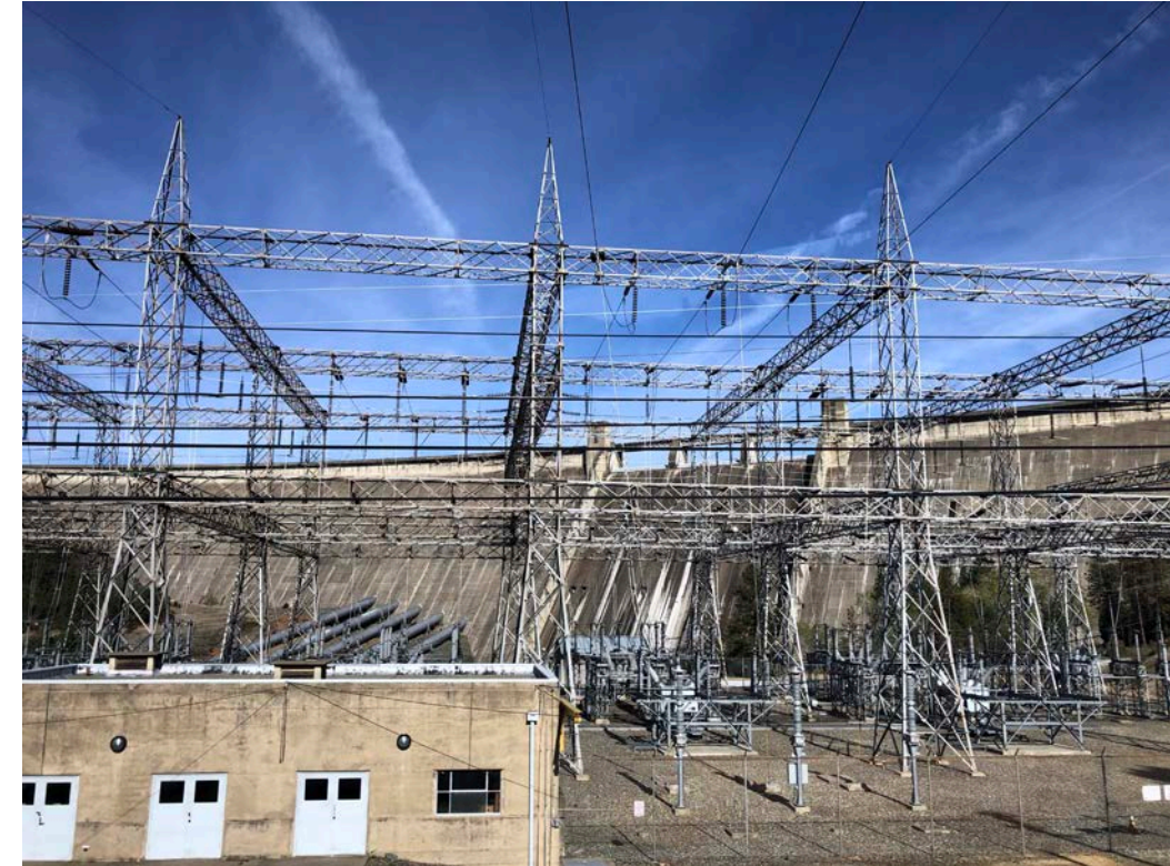
Figure. Hydropower dam substation
