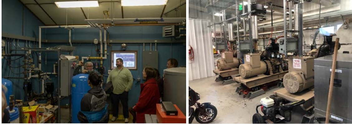
Figure 5. Dave Hostetter led tours of the water filtration plant (left) and power plant with its three diesel generators (right). Photos by Greg Stark (left) and Rebecca Green (right), NREL
